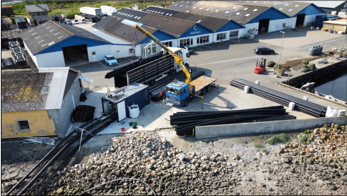
Figure 11: The mussel production units were constructed at the harbour of Hvalpsund, where the pipes were welded on land, and the net mounted when the pipes was pushed out in the water from the welding station. All processes were carried on in a container.
